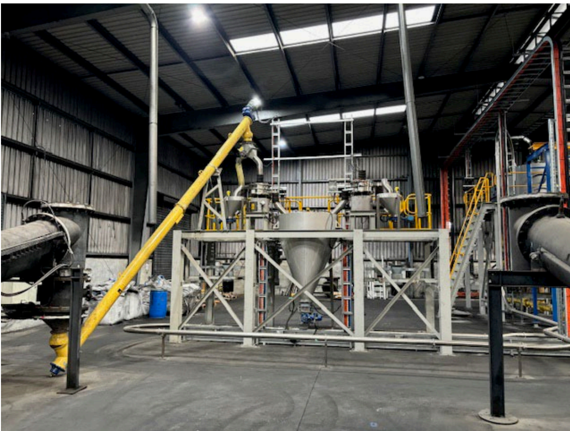
Milling & bagging unit at the Stapylton facility
