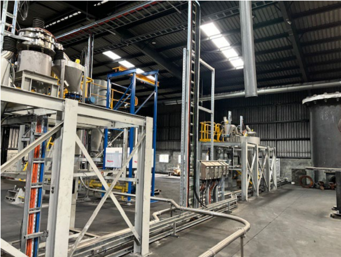
Milling & bagging unit at the Stapylton facility
