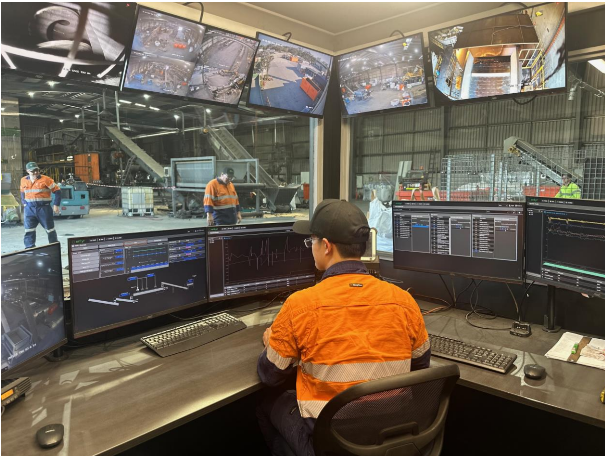
Stapylton control room – upgraded DCS running TDU4
