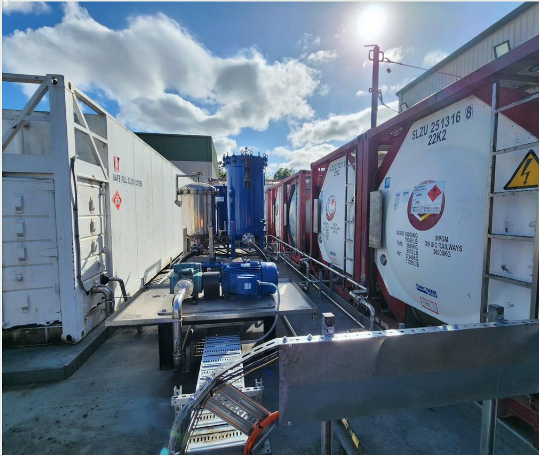
TDFO storage tank farm Entyr's Stapylton site
