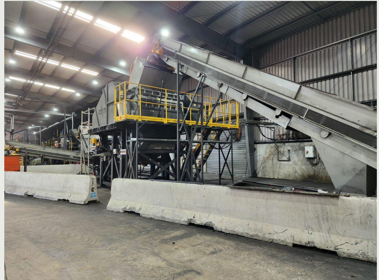
Rasper unit Entyr's Stapylton site
