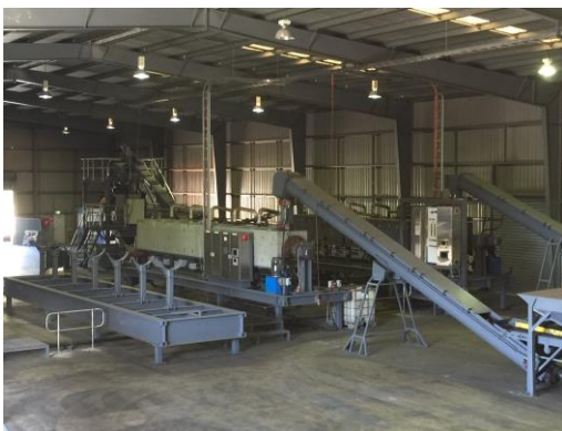
TDUs in operation at Stapylton
